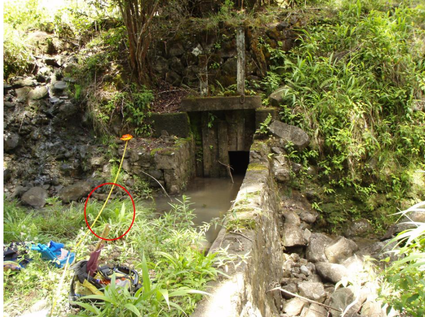
Figure 5-15. Photo of top of the diversion and showing the location of survey site 2 (red circle) and where the flow data was taken. (6/30/2009; Tributary name: Nua'ailua (64010001); PBN: ln002p-002-063009; Surveyor: Kuamo'o, D.; SBN: dk002d-063009; Lat. (DD): 20.83374, Long. (DD): -156.17751).
